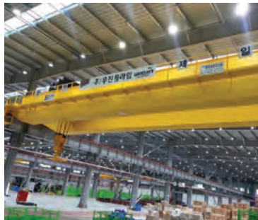
O/H Crane 50Ton SPAN : 30m
