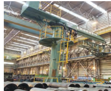
JIB Crane 5Ton JIB-post 6m ARM 12m 360°
