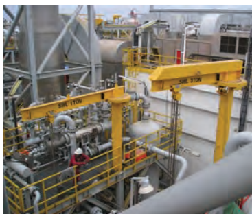
JIB Crane 1Ton JIB-post 3m ARM 3m 270°
