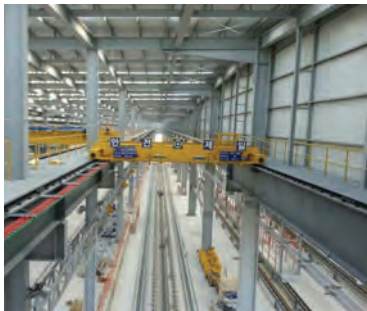
O/H Crane 15Ton SPAN : 15m
